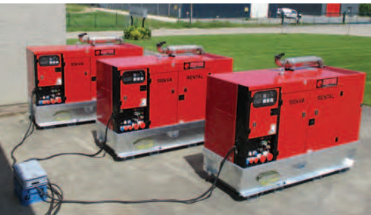
Belgian rental company Delta Rent has been using Europower EPSR rental generators with Volvo engines and in parallel configuration.
